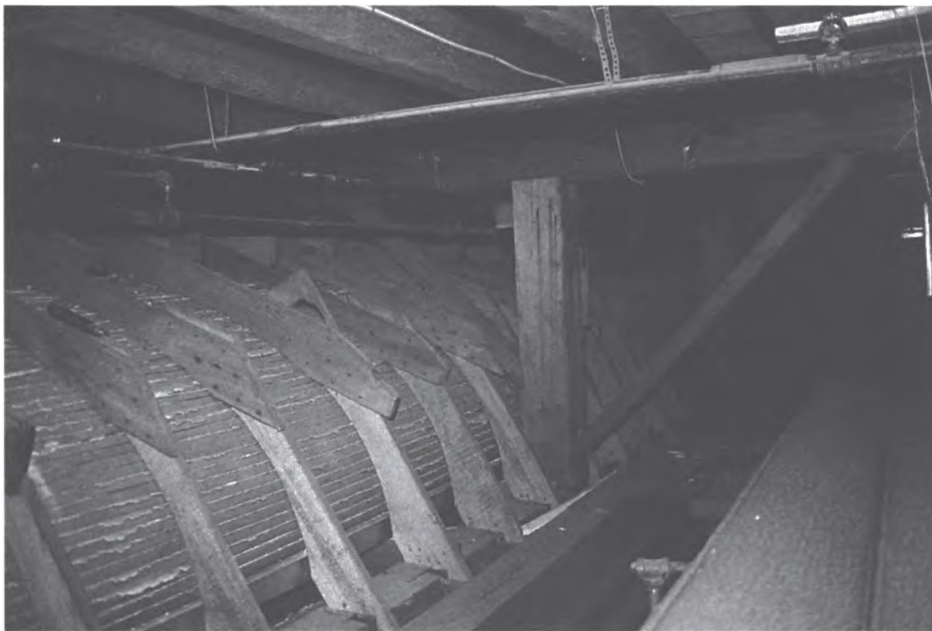
4-4. Detail of structure showing knee braces supporting the girders under the upper-court floor. The photograph was taken in the interstitial space between the ceiling of the lower court and the floor of the upper court. Note the framing for the elliptical ceiling on the left of the photograph. Modern items include stacks of upholstered pads for the wooden benches (lower right), piping for the sprinkler system, and an iron tie rod that was inserted to keep the west wall of the temple from leaning outward.
